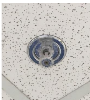
Photograph 5: Sprinkler head covered with lint.
