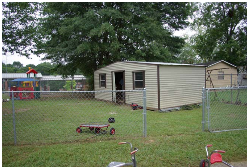
Photograph 10 – Taken at LaGrange on 8/20/2009, showing a playground fence gate off its hinges, allowing children to enter an area where they could access an unlocked storage shed. The gate is propped against the fence.
