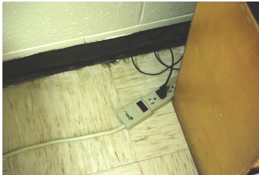
Photograph 6 – Taken at Newnan on 8/18/2009, showing a classroom power strip containing several outlets without protective caps.
