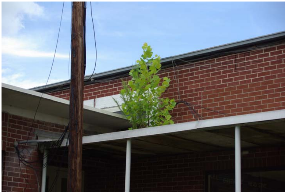
Photograph 2 – Taken at Greenville on 8/18/2009, showing the roof over an outdoor walkway. The roof was leaking, leaving the concrete walkway wet and slippery. The roof had a small tree growing on it and appeared unstable.
