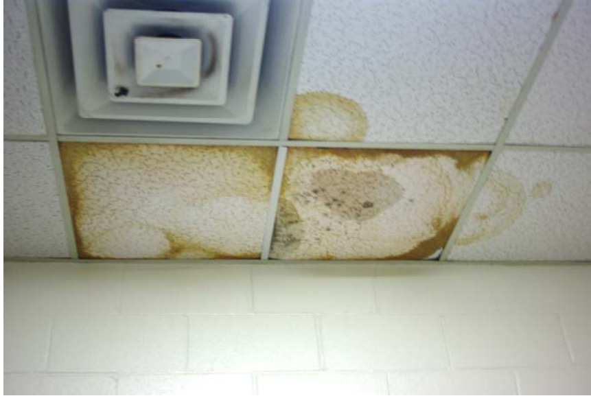
Photograph 5 – Taken at Verona Rosser on 8/18/2009, showing sagging, water-stained, and apparently moldy ceiling tiles.
