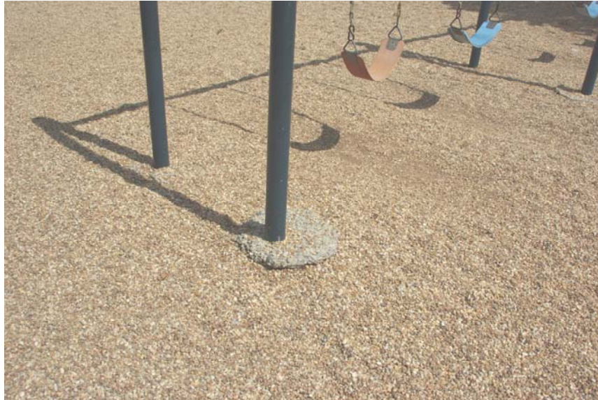
Photograph 7 – Taken at Pine Ridge on 8/19/2009, showing raised concrete at the base of playground equipment.
